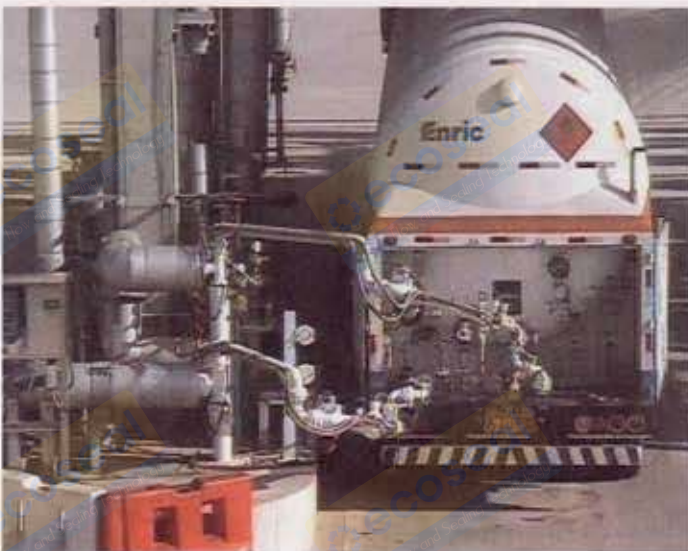
on spot loading facilities
