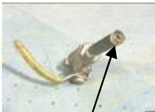
Plugged injection port piping
